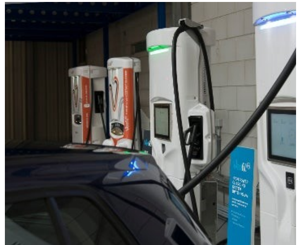
Tritium's electric vehicle charging stations.
