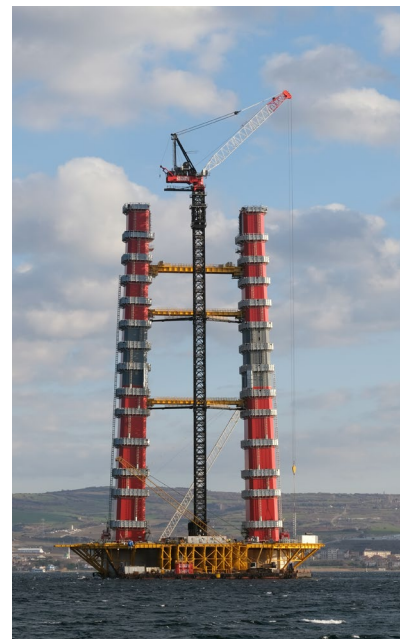
Marr’s M2480D HLL cranes working on the 1915 Çanakkale Bridge across the Dardanelles in Turkey.
